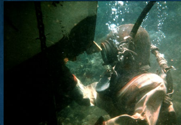
THE PALOMBARO FROM MESSINA AT WORK ON THE YACHT'S DAMAGED STERN. HE IS HAMMERING CHUNKS OF WOOD INTO THE GAPS INTO HOLES TORN IN THE HULL'S STEEL PLATES. EXPERT DIVERS WILL APPRECIATE SUCH LOCAL MAINTENANCE HABITS, WHILE PERHAPS STUDYING THE FINE REPAIR JOB ON THE PALOMBARO'S OWN HELMET AND FITTINGS.
